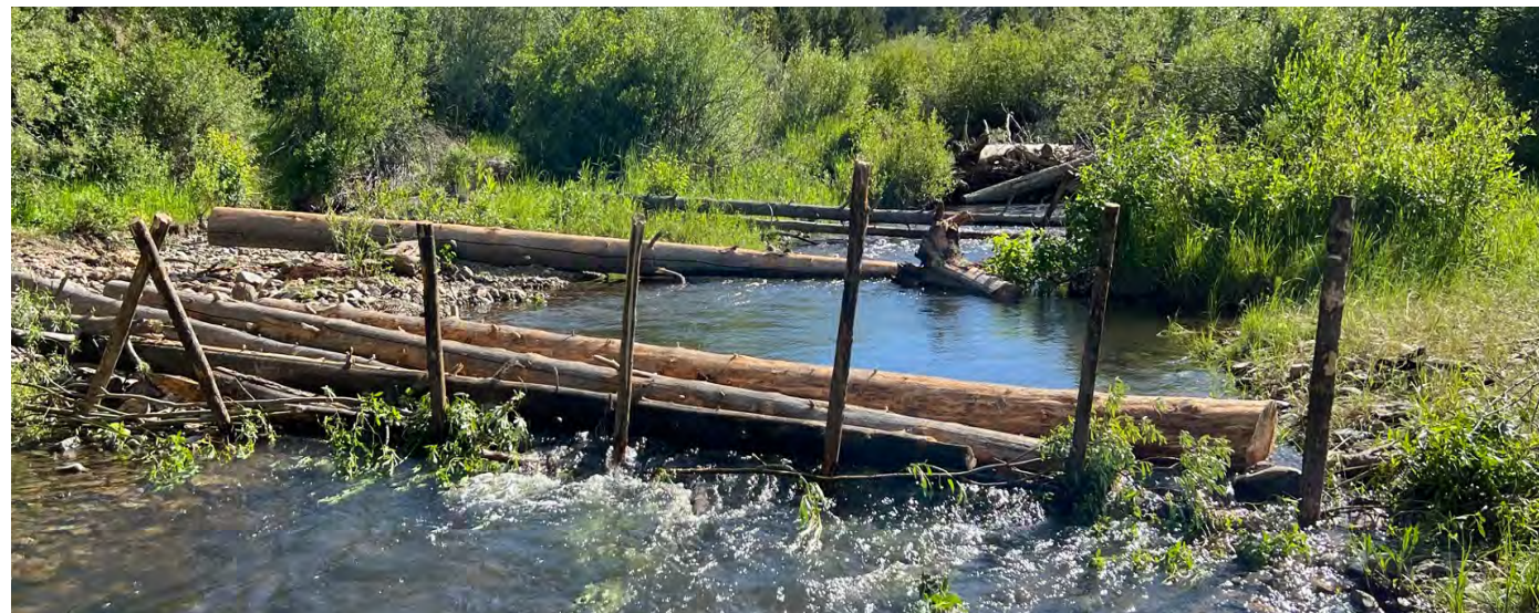
Panther Creek, example of a Post Assisted Log Structure. Photo taken July 15, 2022 (credit: Boyd Bouwes, Watershed Solutions, Inc.)
