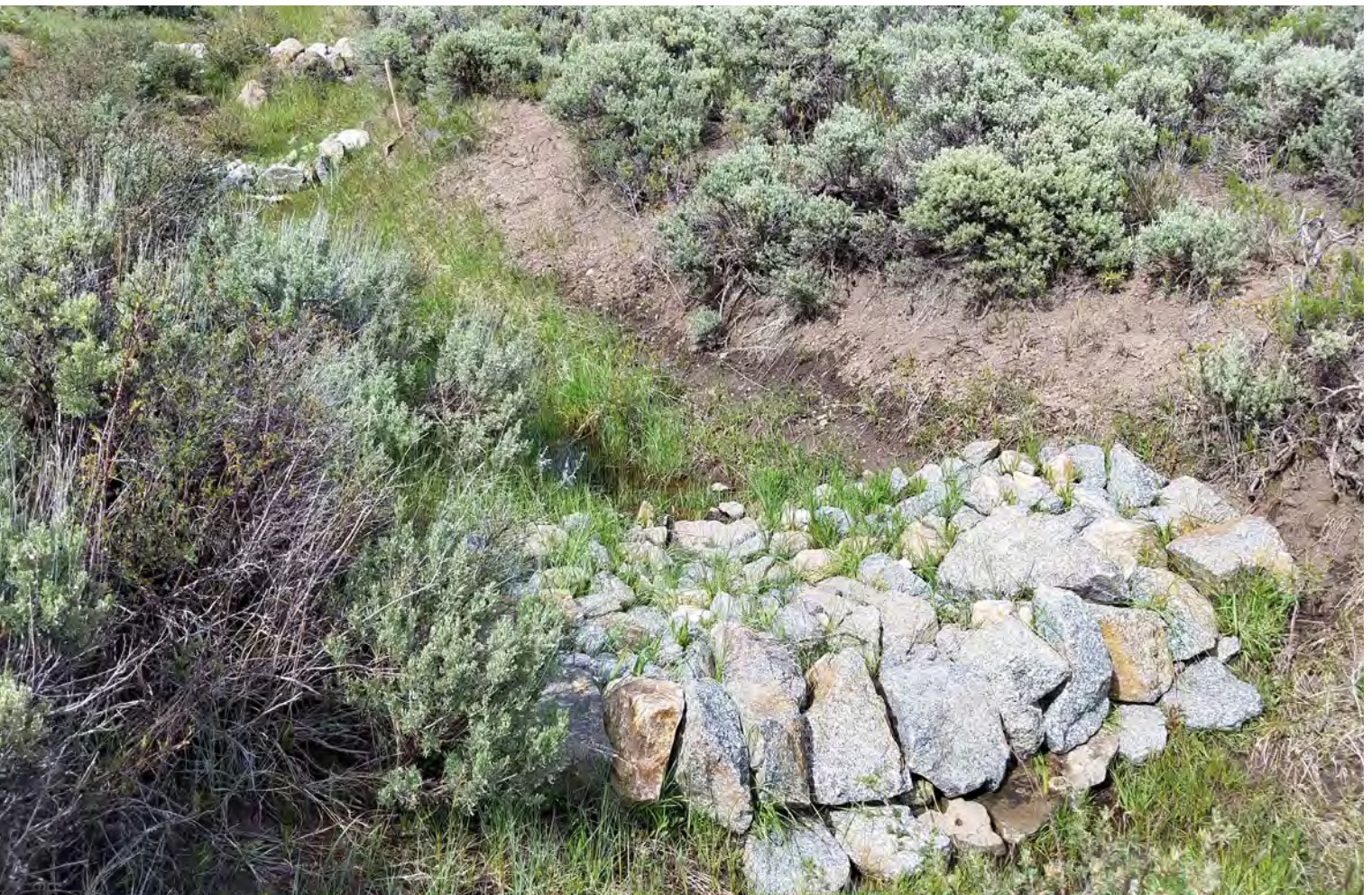
Zeedyk rock structures restoring an incised channel. Photo credit: Nathan Seward, Colorado Parks and Wildlife.
